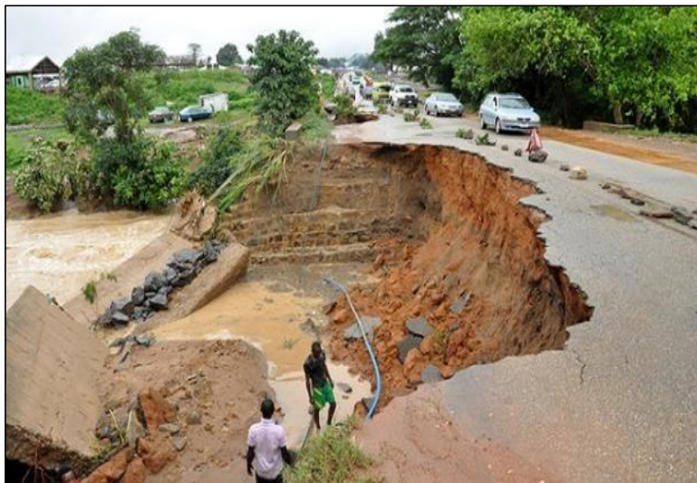
Plate 4: Effects of Flood on Road Pavement
