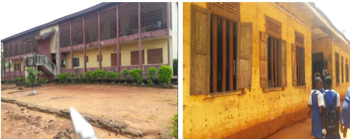
Plate 2: Showing dilapidated classroom blocks in the schools in the study area.
