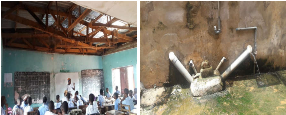
Plate 1: Showing classroom without ceiling boards and dilapidated sanitary fittings in a school building
