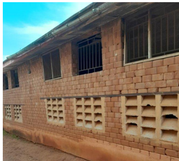
(b) ICEB classroom — permanent screen wall ventilation
